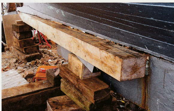
Clockwise from top left: the new laminated stem; replanking the coachroof; three-metre length of oak for the keel being lifted into position
